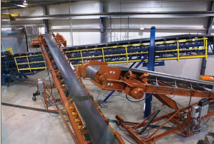
At the Center for Innovation, the process simulation area incorporates a three-belt recirculating conveyor loop carrying materials for observation of material flow and component life.
